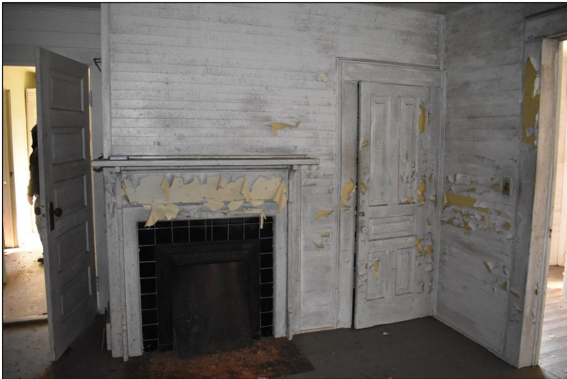
Figure 15: Fireplace, five-paneled door, surrounds, and wallboards in first story of original block.
