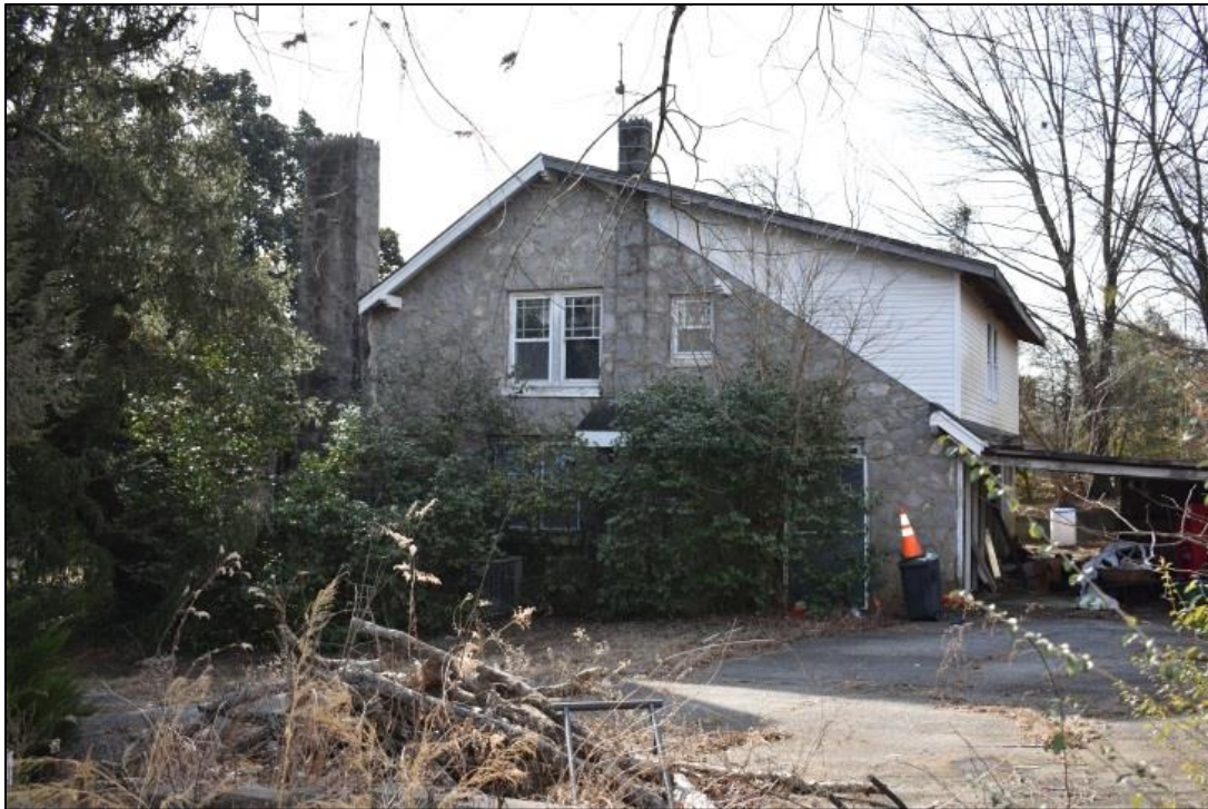
Figure 37: View of side (northern) elevation of Ledford House with later-added shed dormer rising at rear.
