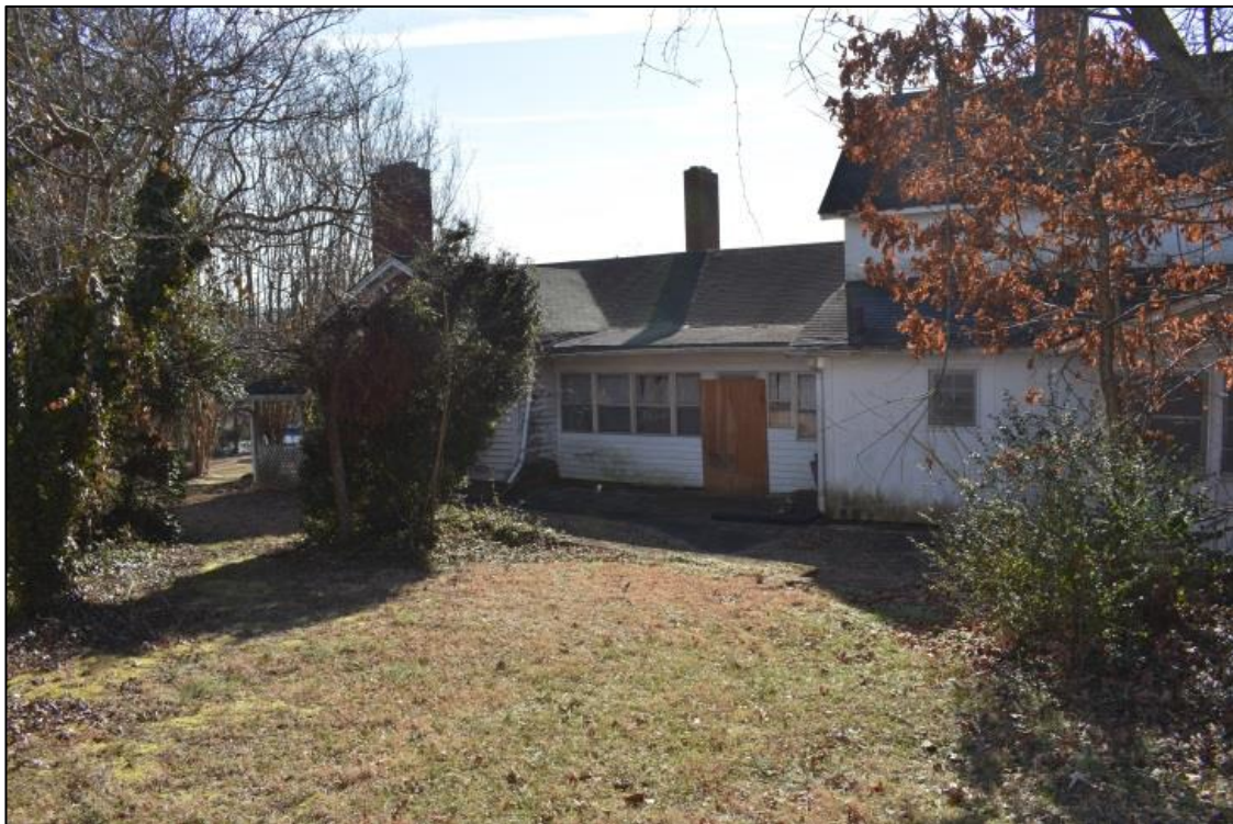
Figure 13: View of (northern) rear elevation of hyphen with once-open porch converted into sunroom.
