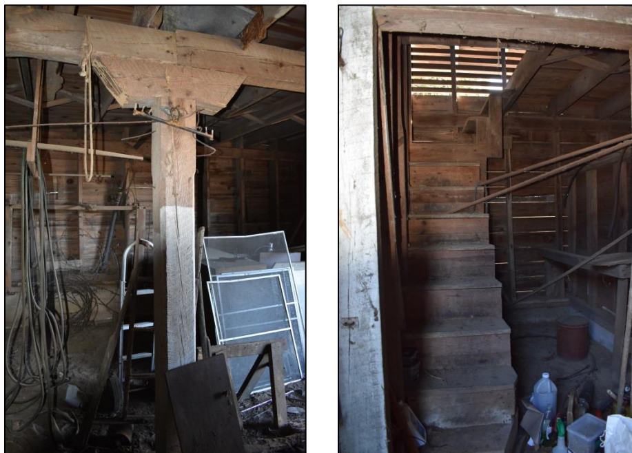
Figure 30: Left, interior view of barn looking to east; right, view of staircase to second floor, located in the barn's southeastern corner.
